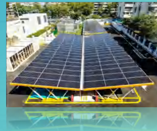
120KWP PV canopy
